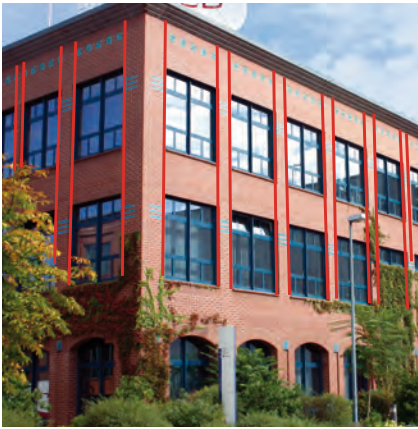
Continuous vertical expansion joints next to openings (horizontal expansion joints not shown)
