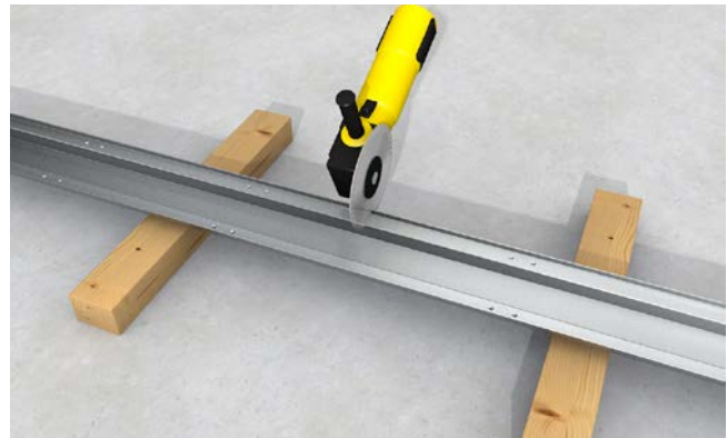
Cut the trunking segments and cover to size and check the fit in the milling zone.
