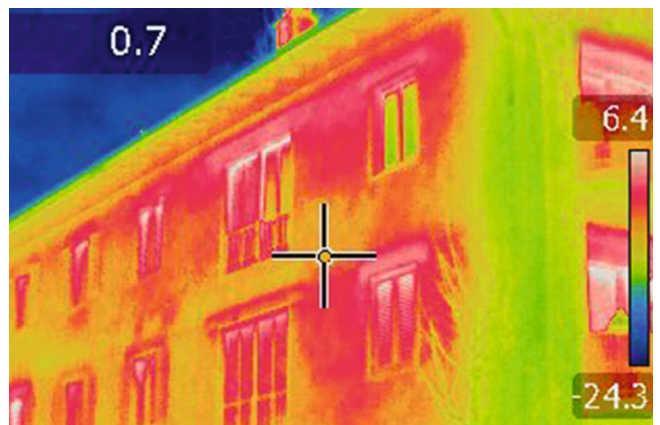
Visualisation of thermal bridges by means of thermography
