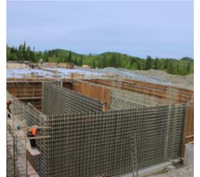
Tanks for sewage treatment plant, wall and floor slab reinforcement Thetford Mines, Québec, Canada
