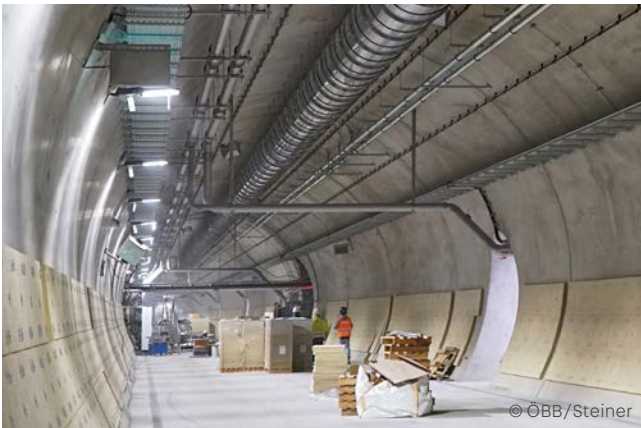
Supply tunnel, Koralm Tunnel (Carinthia / Styria, Austria)
