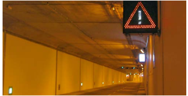
Lighting and signalling systems
