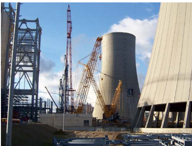
Neurath power plant in Grevenbroich, Germany
