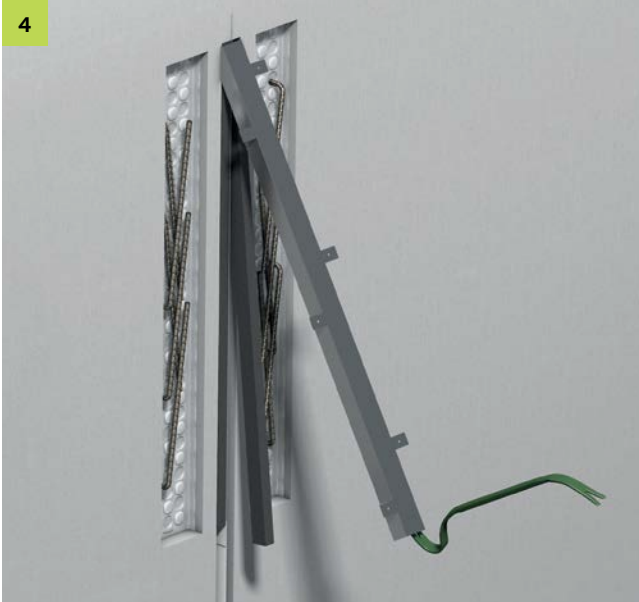
After casting the first section, remove the protective boxes of the FERBOX® rebend connectors, the protective boxes of the PENTAFLEX® Modul and the EPP filling strips.
