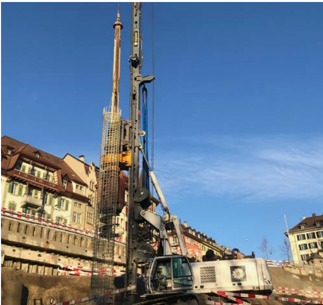
Bored piles in the Wildpark excavation pit Future train station, Bern, Switzerland
