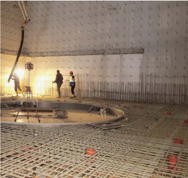
Ground slab and column reinforcement as well as punching shear reinforcement Fusion energy research project Tokamak in Prague, Czech Republic
