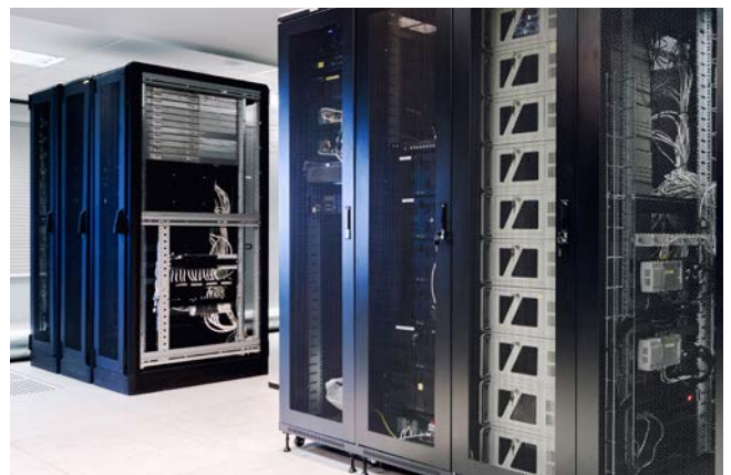
Server cabinets and racks hold hardware securely in place and ensure they are able to operate properly.
