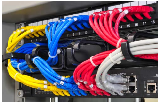
Orderly cabling improves system efficiency: diagnostics and maintenance become easier and heat dissipation is improved.
